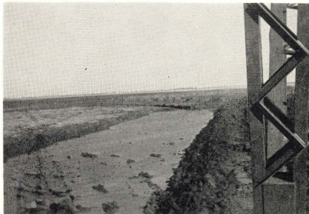
Barrow pit for dikes in Cheyenne Bottoms. This picture was taken in January by F. Sharon Foster, resident engineer on the Cheyenne Bottoms project.
